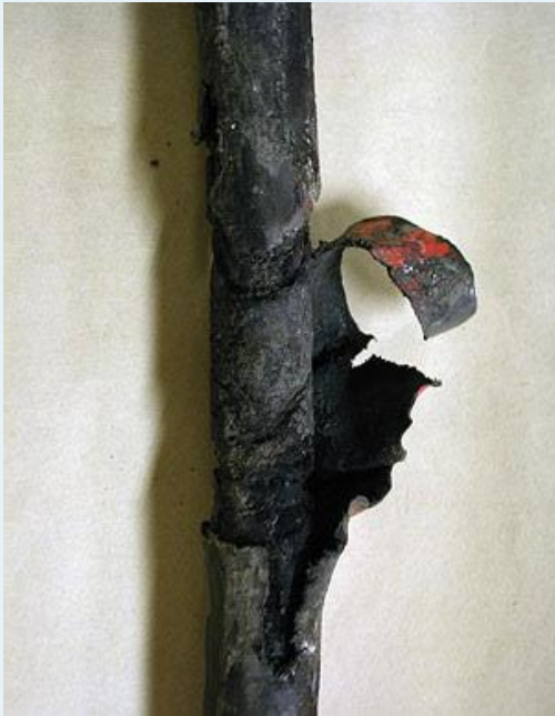
Failing electricity cable/joint
